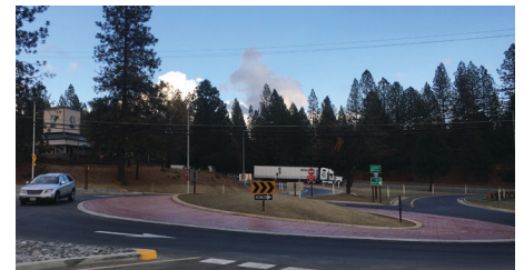
- Creation of a Roundabout in Colfax between Auburn Street and the I-80 Ramps
