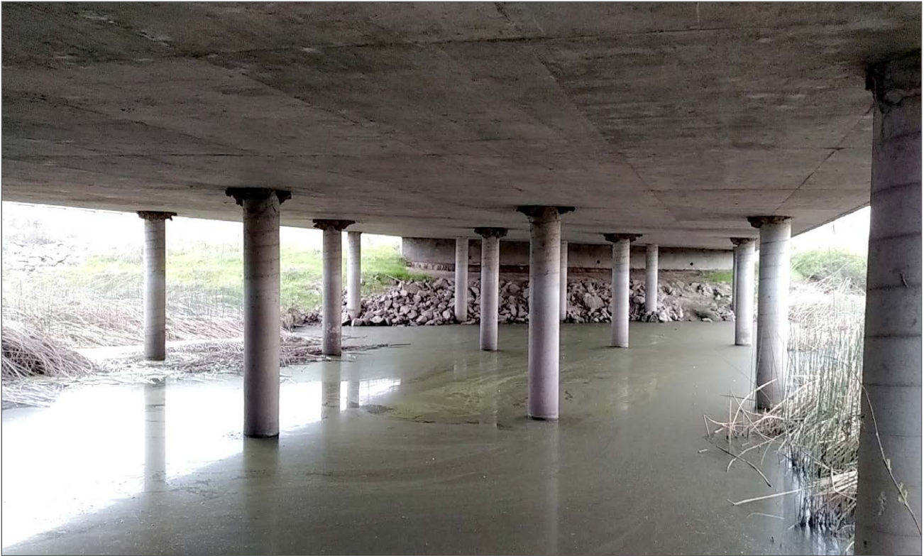
Photo 5: Remnant swallow nests on underside of southbound SR 65 bridge over Pleasant Grove Creek (facing south; 2/05/15)
