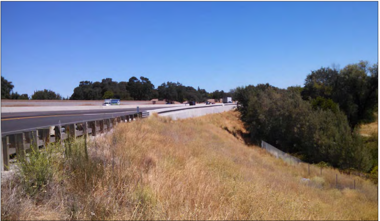
Photo 5: Proposed encroachment area for Secret Ravine northeast of the I-80/SR 65 connector ramp (facing northeast; 7/23/14)
