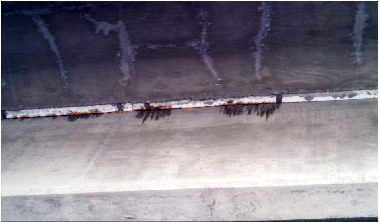
Photo 1: Bat urine staining underneath the existing I-80 deck structure over Miners Ravine (7/23/14)
